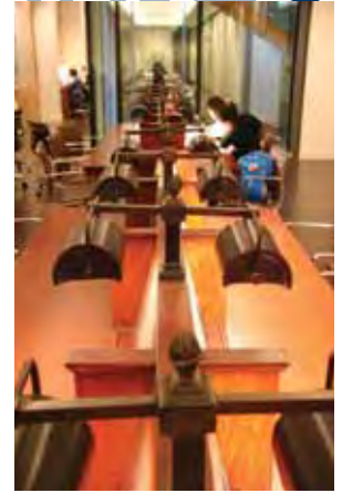
UCB Refurbished existing carrell lights
